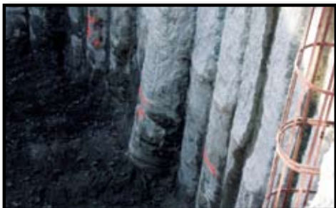
Picture 1 - The anomaly shown here was not remedied prior to concrete placement to assure verticality. All other piles on this project were constructed to within 0.1% of verticality.
